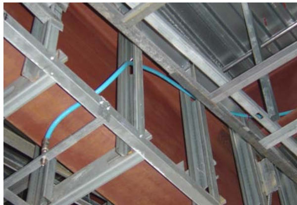
Plenum Cable Detail (installed in ceiling)
